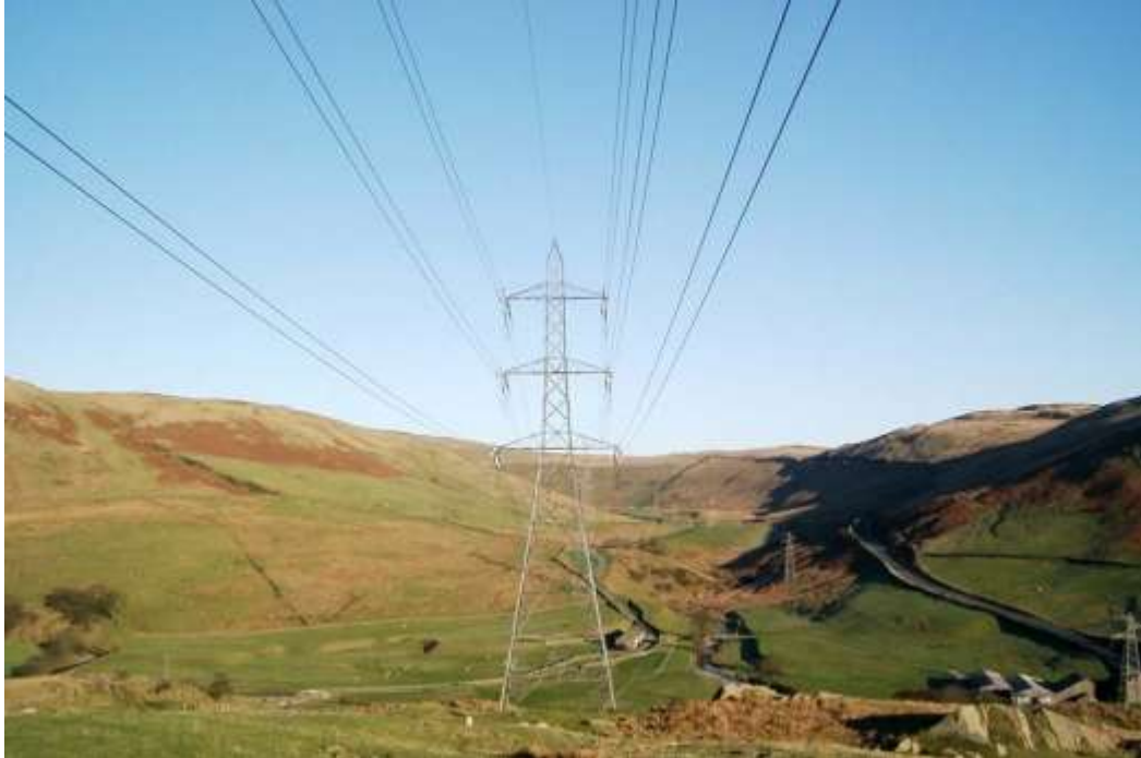
Pylons in the Lake District
